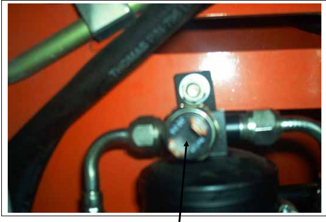
Binary pressure switch on receiver drier. One terminal goes to the compressor and the other goes to the A/C unit.
