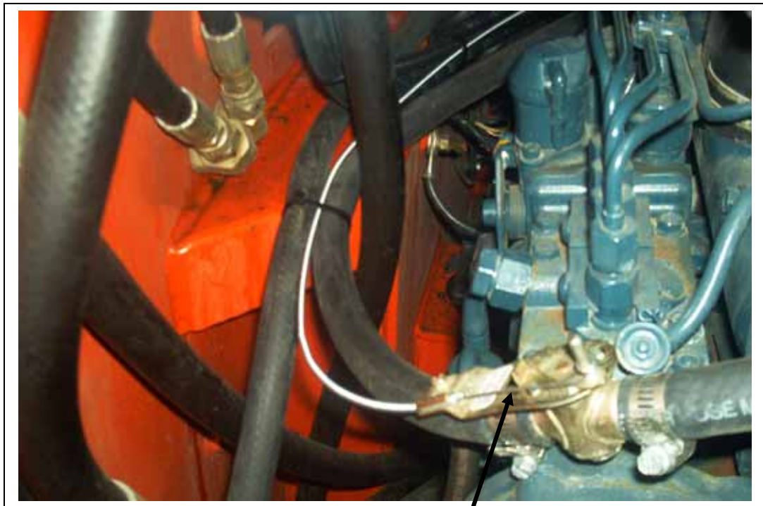
Cable controlled heater shut valve.
