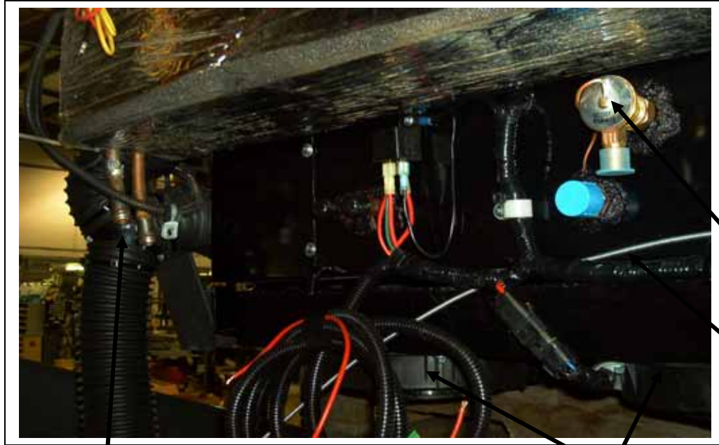
Heater line connections
