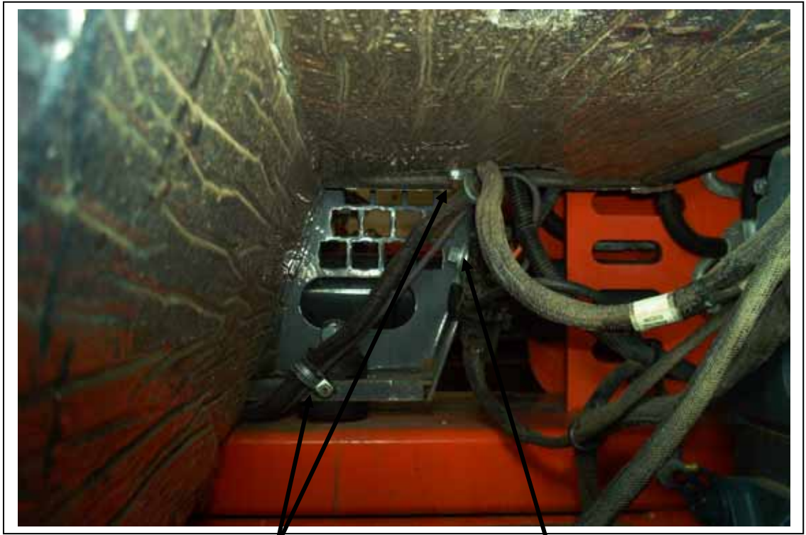
"P" clamps holding wire harness
